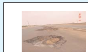
Photo 5: Pavement Premature Failure
